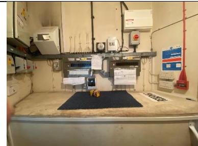
Figure 36 Example of switchgear
