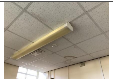
Figure 39 Example of fluorescent lighting
