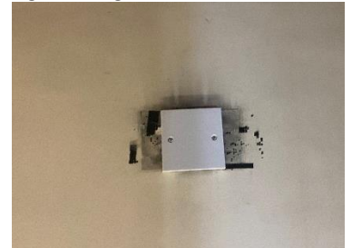
Figure 38 Failed socket outlet
