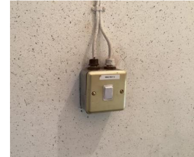
Figure 37 Light switch with MICC feed
